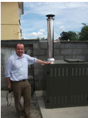
Mr Liam Fleming- Energy Manager Waterford Co Council, Ireland at a Outdoor Pellet boiler in Co Waterford
