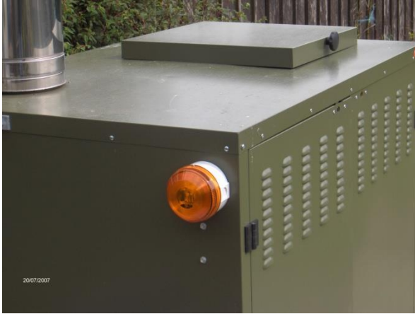
Low Level Fuel Warning light
